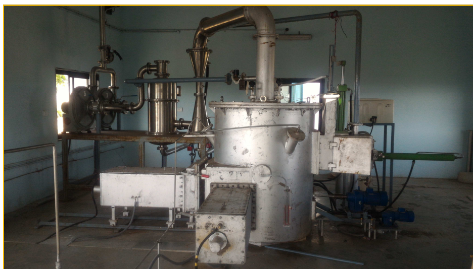
Plasma Pyrolysis / Gasification System installed at CSIR- CSMCRI
